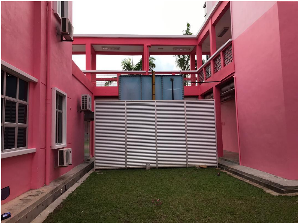
Rainwater Harvesting System in School of Microelectronic Engineering Building
