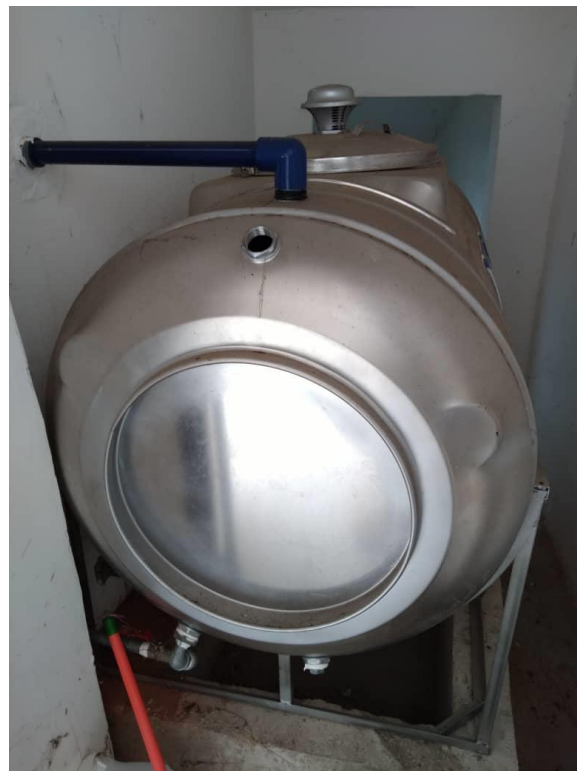
Rainwater Harvesting System in Digital Management and Development Centre (DMDC) Building
