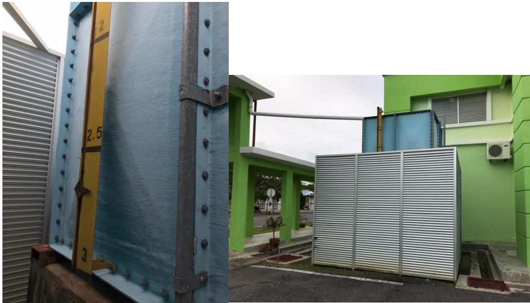
Rainwater Harvesting System in Engineering Centre Building
